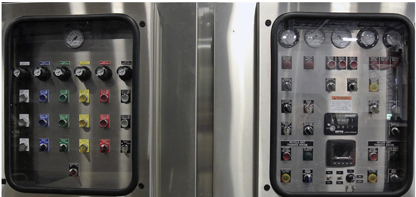
Adequately designed, low voltage (24vdc and lower) control panels are the safest systems for mobile use.
